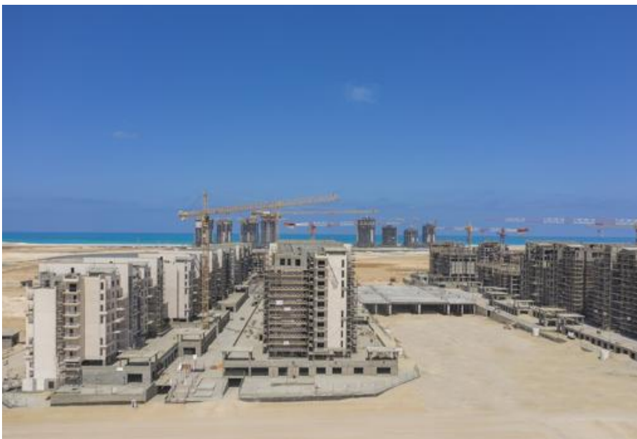
An enormous residential complex currently being built in Egypt, for which MPLifts has supplied 112 lifts for a value of 1.5 million euros – ABC
